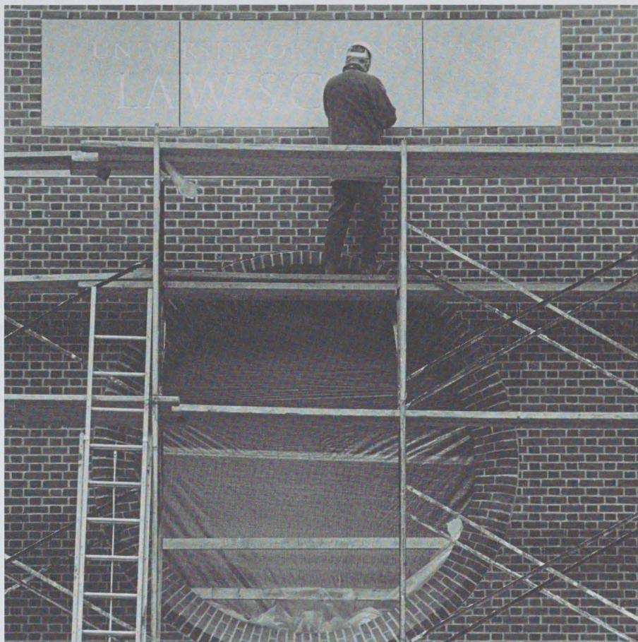
Master stone cutter Richard Grasby inscribes the stonework over the Law School's new main entrance in the south side of Nicole E. Tanenbaum Hall.
