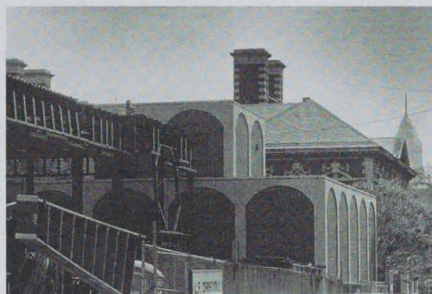
In May, 1992, steelworkers lifted the last beam and topped off the building. This view is taken from the west end of Sansom Street, looking east toward Lewis Hall.
